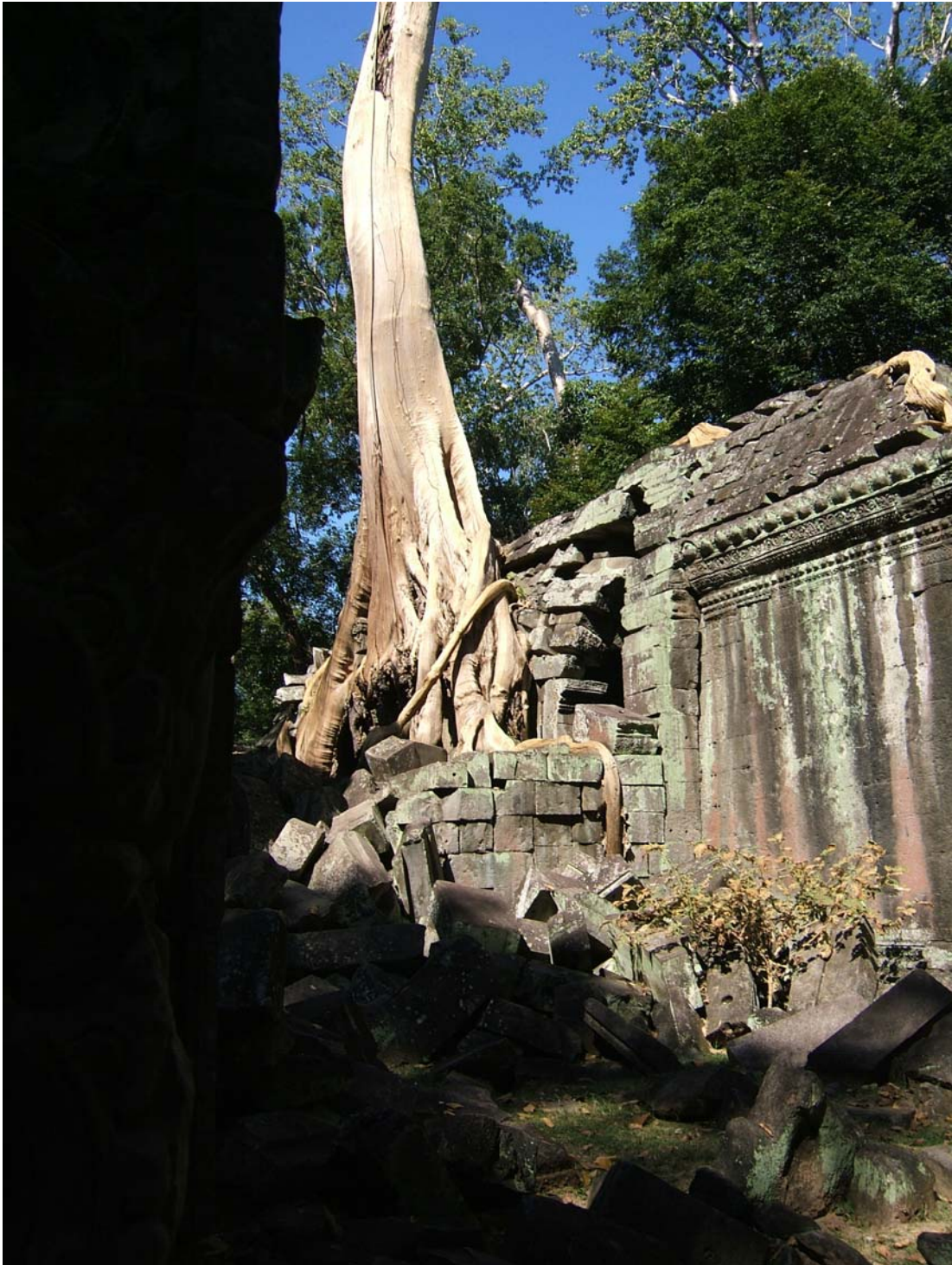
Figure 5-11. At Ta Prohm, the giant trees of the Angkor forest consume the ruins, whilst at the same time holding the structures together.
