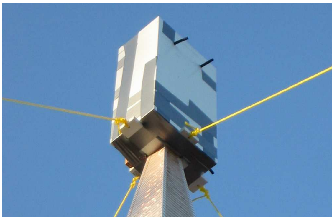
Fig. 5.3: LNA box fitted at antenna apex.
