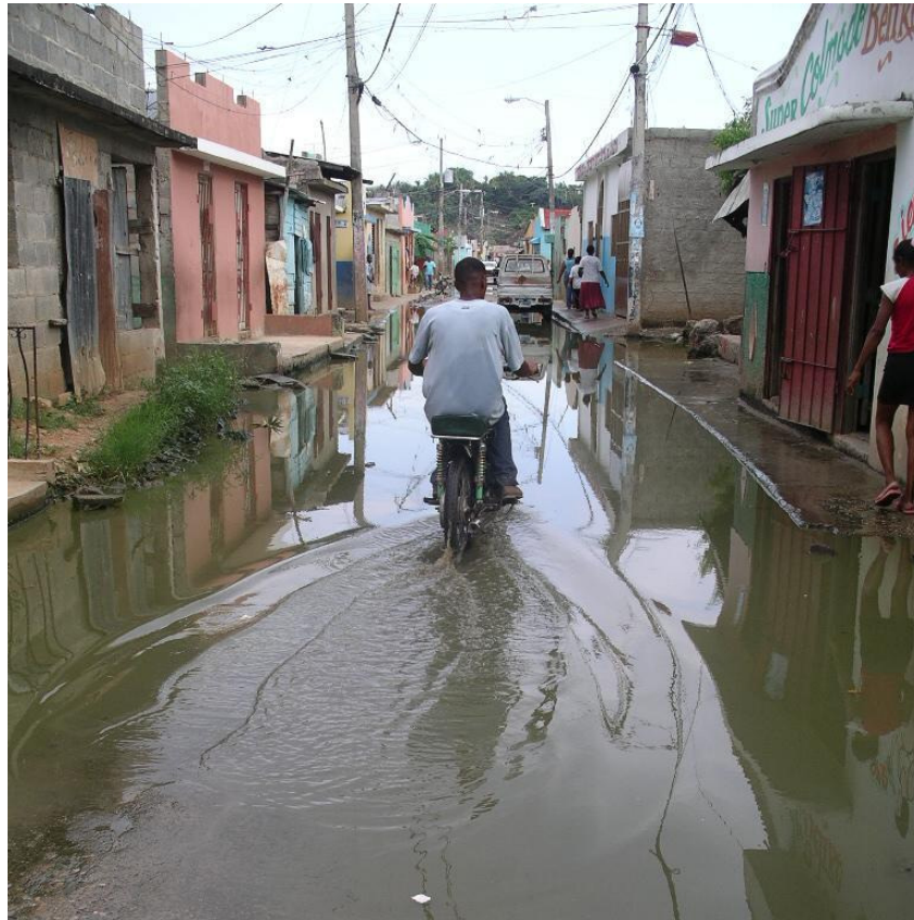
Figure 9. Calle Nueve in the dry season before stormwater drains were installed in La Ciénaga.
