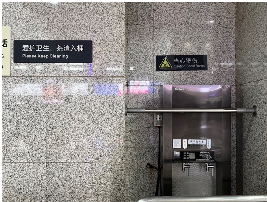
Figure 6. 15: A hot water area
