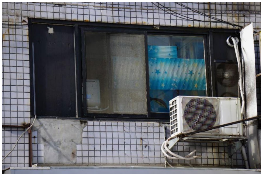
Figure 1.2 Tiles fall off from an old residential building [34]
