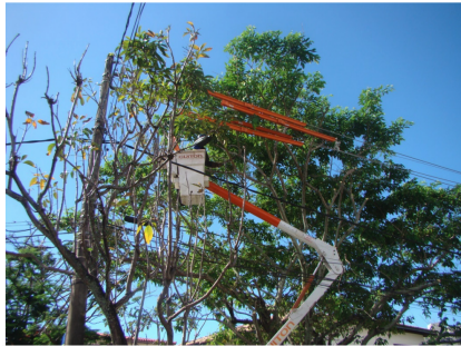
(a) Manual pruning of overhanging branches impeding power lines, from Siebert et al. (2014).
