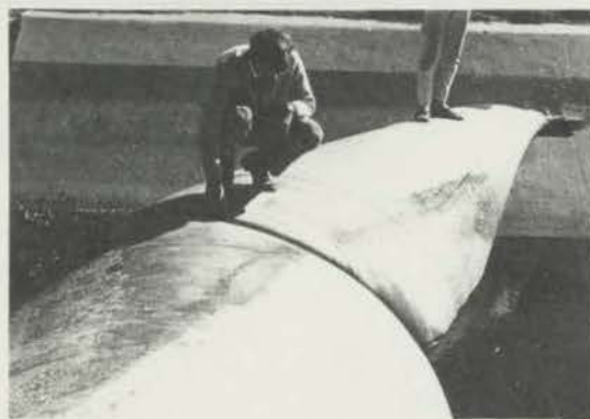
DIAGRAM 3.14 - THE LARGE CREASES AT THE ENDS OF THE FABRIDAMS. STRESSES ARE PROBABLY DECREASED IN THE CREASE, BUT INCREASED ON THE OTHER SIDE. ALTHOUGH THE BAG APPEARS OVER-INFLATED AT PRESENT WATER MARKS INDICATE EFFICIENCY OF DAM AT HIGH TIDES.
