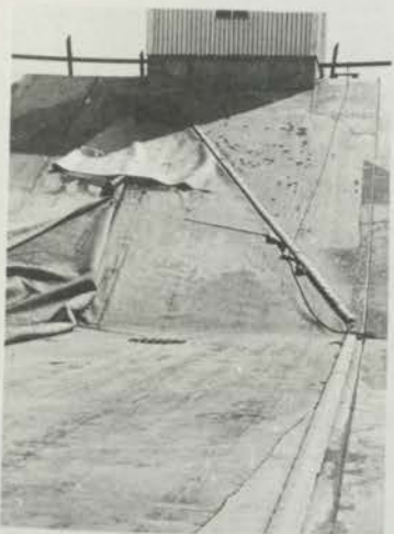
DIAGRAM 3.25 - A VIEW OF FAILURE SHOWING RIPPED FABRIC. FAILURE APPEARED TO HAVE BEEN INITIATED AT RIGHT CORNER OF CLAMP LINES.
