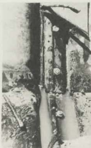
DIAGRAM 3.34 - A VIEW OF SECTION WHERE FABRIC PULLED AND INTERNAL TUBE WHICH HAS PULLED OUT FROM UNDER THE CLAMP.
