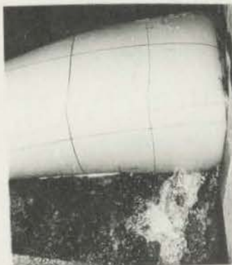
DIAGRAM 5.21 - TUCKED IN END IN AIR-INFLATED DAM, NOTE THE LEAKAGE AROUND THE END.
