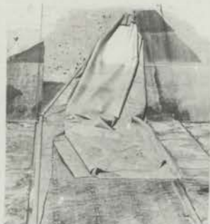
DIAGRAM 3.26 - TEAR APPEARED TO PROCEED ALONG BASE CLAMP FOR MORE THAN 100 FT, THEN RUN TRANSVERSELY UNTIL UPSTREAM HEAD LOWERED.
