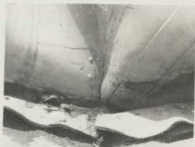
DIAGRAM 3.32 - THE LEFT HAND DOWNSTREAM CORNER - OBSERVE THE CONTORTED FABRIC, A POSSIBLE AREA OF STRESS CONCENTRATION.
