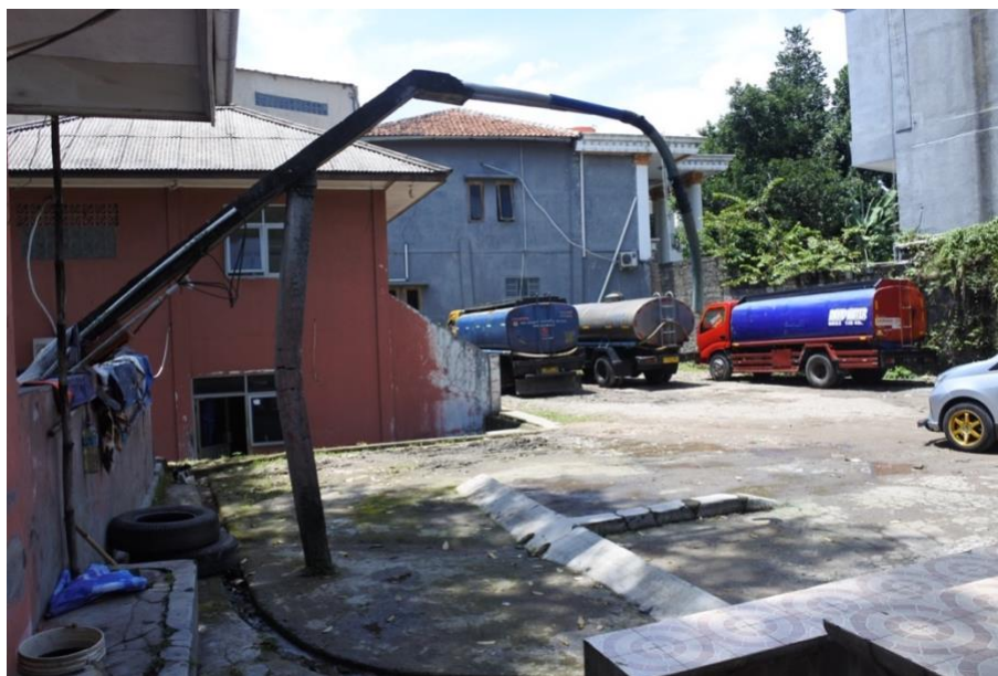
Figure 8.1 Belalai , literally looks like elephant’s trunk, to channel water into the tankers
