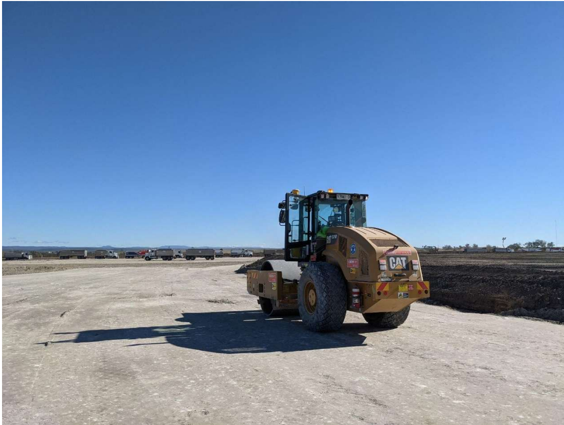
Figure 4-2: Instrumented roller at the project, note the GPS and digital monitors attached to the cab (20/4/21)
