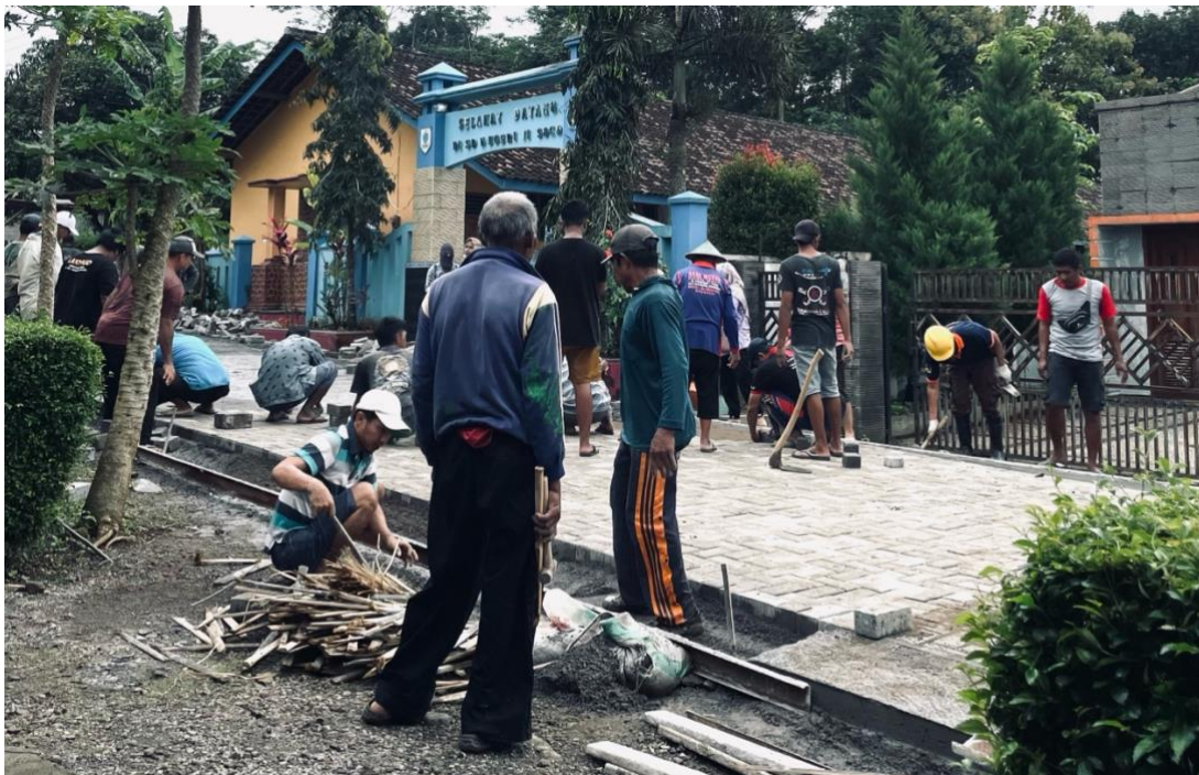
Figure 10: Road Repair in Soco, 27 February 2023
