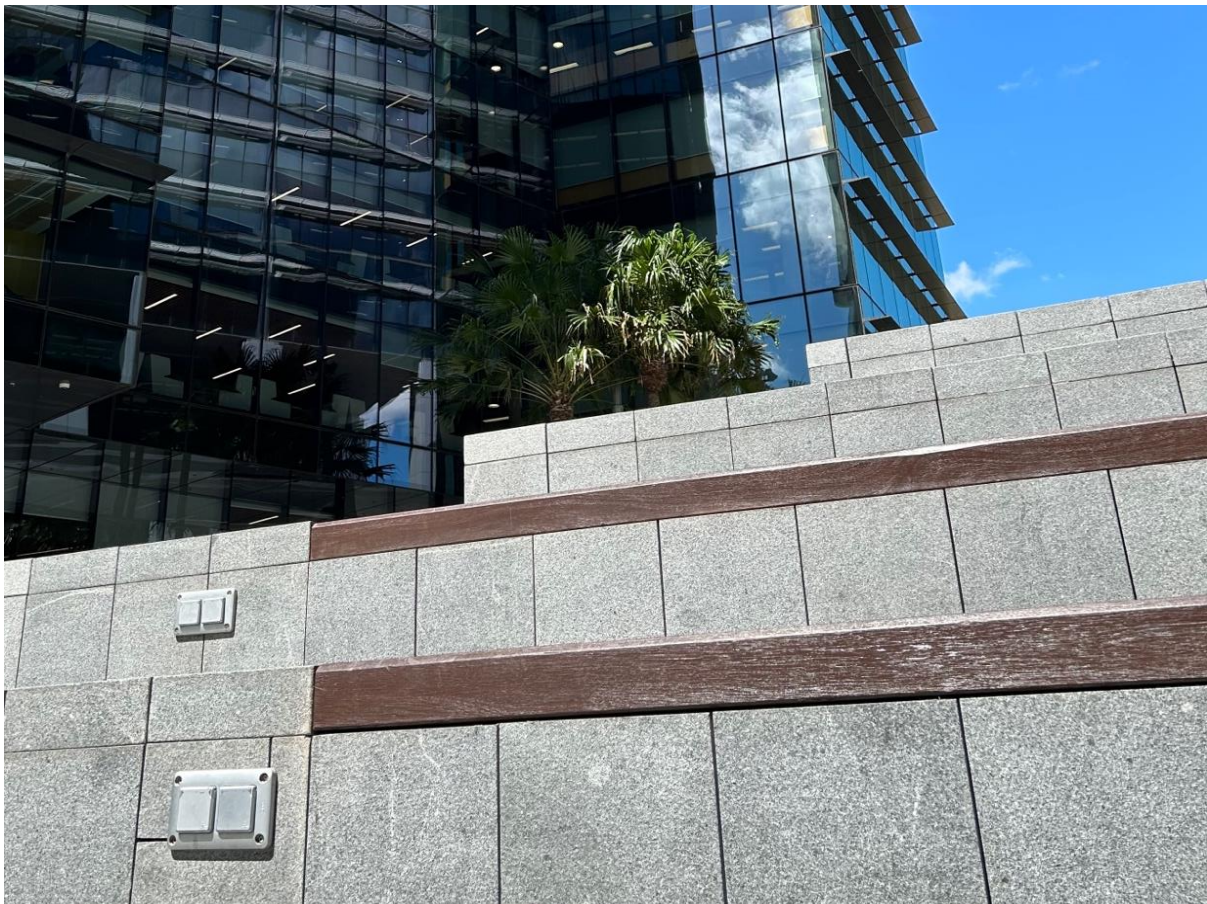
Figure 35 Outdoor charging outlets were installed at IPSQ, City of Parramatta, Sydney, December 2023.
