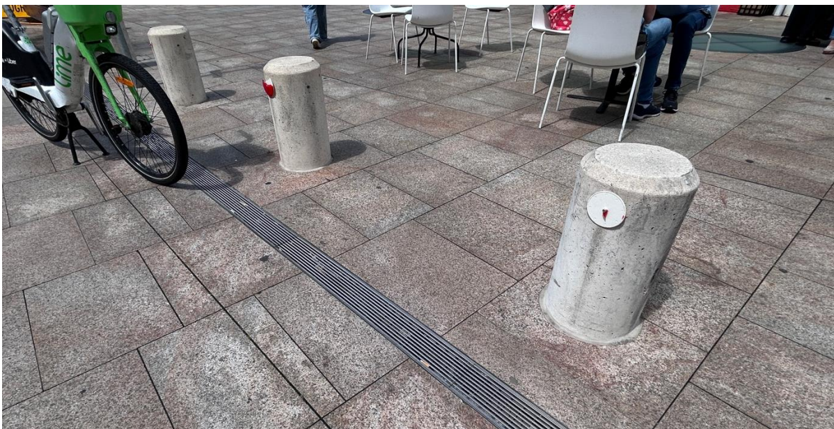
Figure 59 The reflective safety signs on Green Square Plaza were damaged and not visible under some weather conditions, February 2024.
