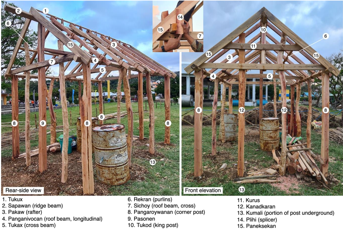
Figure 4.7. The indigenous method of timber construction comes with local names for the parts of the framing system. (Note: The structure shown is constructed for a shed, but the framing system is generic for residential construction.)
