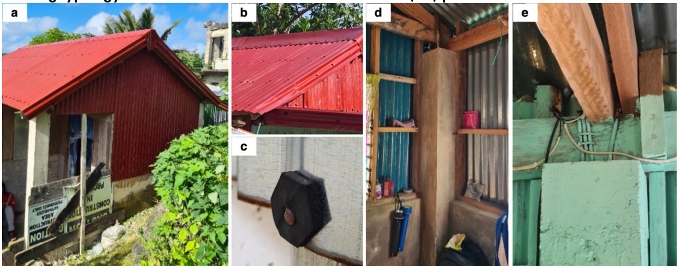
Figure 5. (a) An archetype of a semi-concrete structure with RC posts. (b) Roof/wall sheets are common to be fastened every one or two corrugations. (c) Improvised rubber washers for nail fasteners. Common post and beam connections are (d, e) dowels wrapped around beams and roof members.
