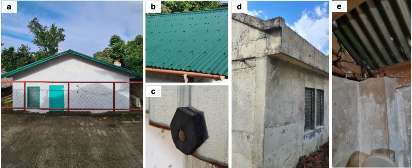
Figure 6. (a) An archetype of a reinforced concrete structure with lightweight roof. (b) Roof sheets are fastened every one or two corrugations. (c) Nails as fasteners come with improvised rubber washers. (d) In some structures, inside gutters are common to conceal the edges of roofing sheets. (e) Roof-to-wall connections are common to be via dowels from reinforcing steel bars wrapping the wooden roof members.
