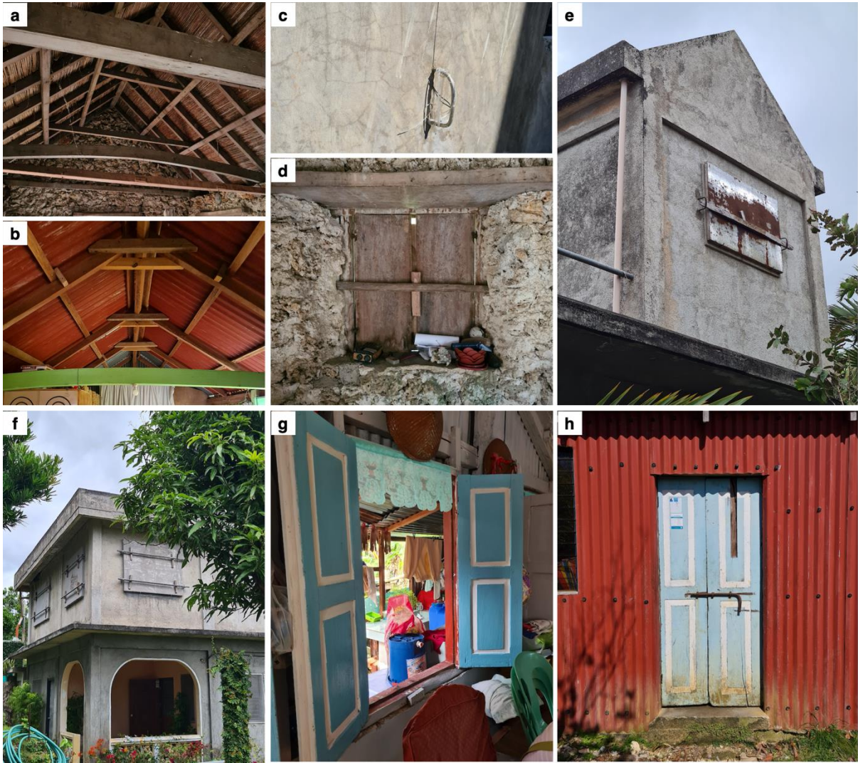
Figure 4.6. Retained construction and typhoon preparedness practices. (a) Indigenous roof framing system of a stone-and-lime house. (b) The indigenous roof framing system as applied to a new housing typology. (c) A steel anchor embedded on a concrete wall of a contemporary house which is used to secure ropes or ties as part of the continued practice of tying houses in preparation for typhoons. (d) From the inside of a vernacular stone-and-lime house, a horizontal bar ( vavangtal ) is used to secure windows and prevent wind and rainwater intrusion. (e, f) This concept has now evolved and is used
