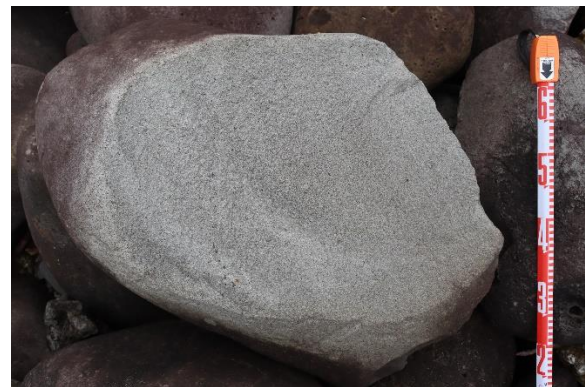
Figure 25: Example of boulder fracturing from machinery or heavy seas. Photograph by N. Jorgensen.
