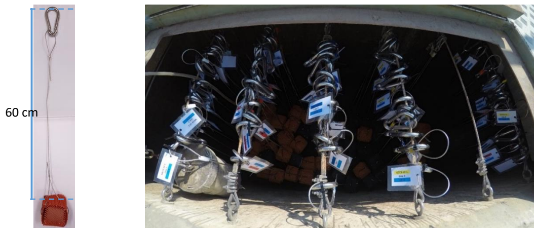
Figure 3-6. Basket with length adjustment (left) and Cube coupons installed on the wires inside an access chamber (right)
