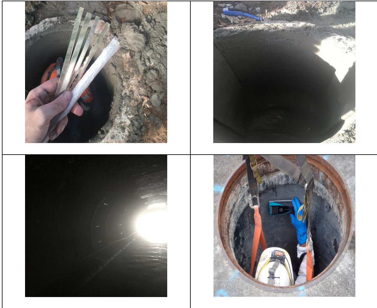
Figure 3-13 Ni-Al alloy rebars (top-left); false rebar installation in access chamber (top-right); false rebar installation in sewer pipe (bottom-left); cover meter testing of coating thickness (bottom-right)
