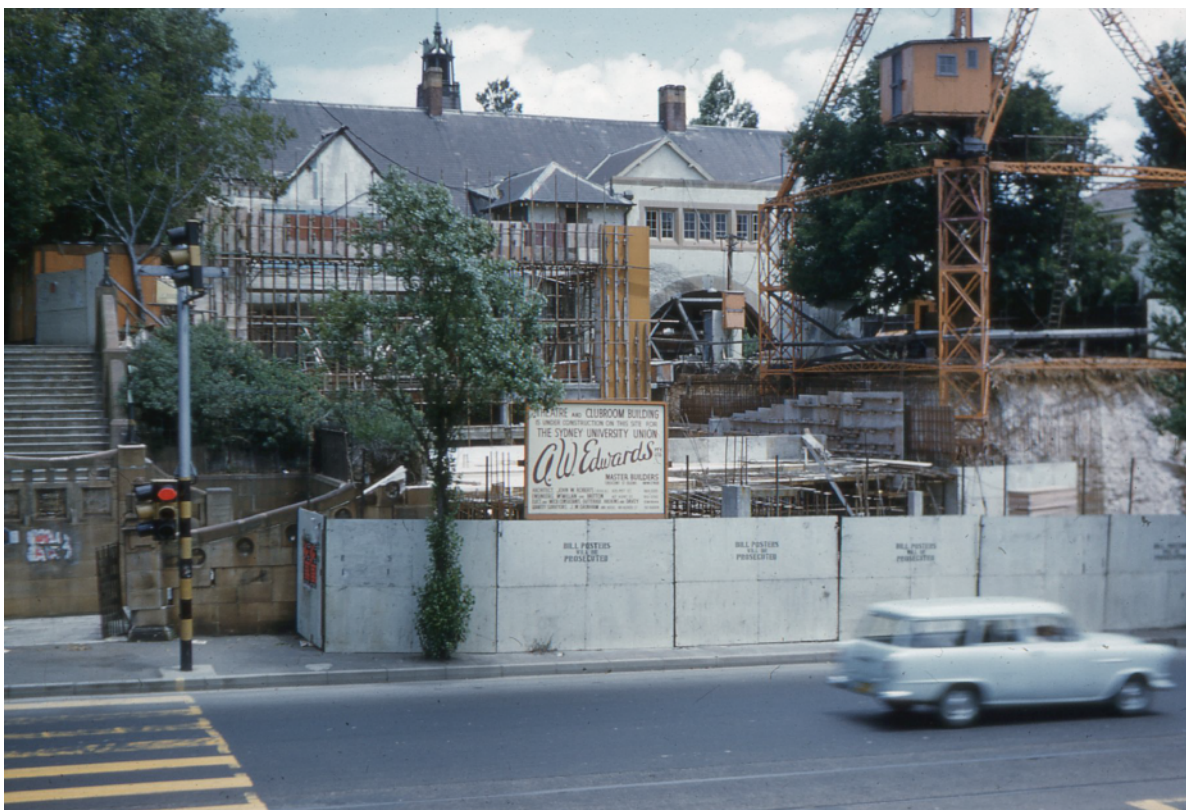
2.21 Work beginning on the site of the old Union Theatre on Parramatta Road 7/1/1961. Was it really a year since the demolition of the old Theatre in the previous photo and the small amount of progress evident in this one?
