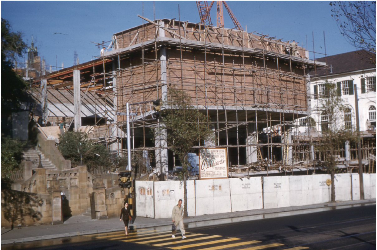
3.10 The new Union Theatre 1/6/1961. Work towards the new theatre was now well under way.
