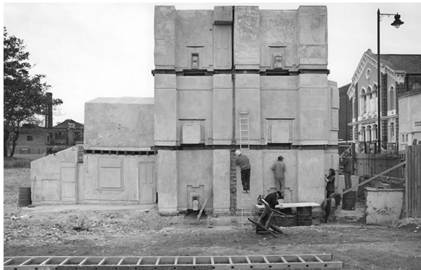
Figure 19 - House (during construction) , Rachel Whiteread, 1993. Commissioned and produced Artangel, London. Image reproduced courtesy Artangel.
