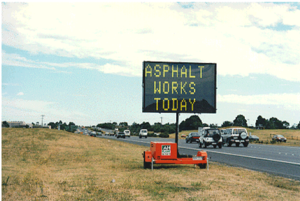
Figure 4: Advance Warning VMS
