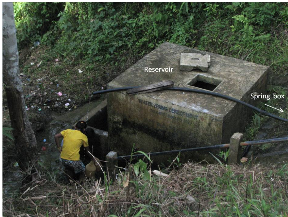
Figure 5.2: The tub, Policarpo's main water source
