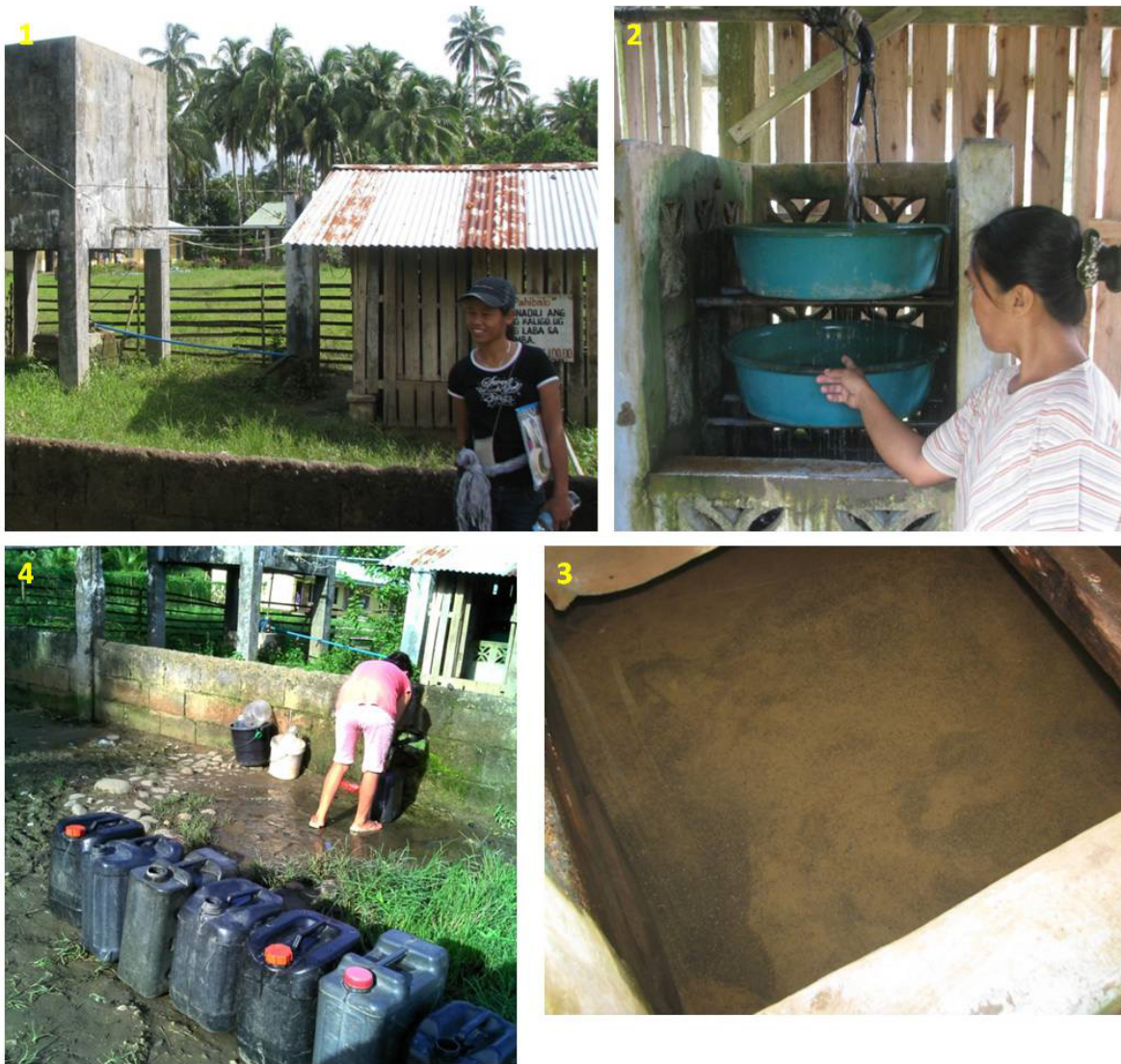
Photo 1: The reserboyr water source, consisting of the tank and the water filter shed; Photo 2: Charcoal basins for iron smell removal; Photo 3: the sediment filter; Photo 4: Water outlet
