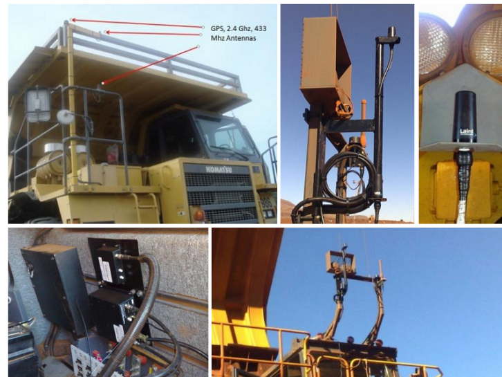
Figure 1.3 – Wireless communication devices mounted on a vehicle. The figure shows the installation of radio transceivers and associated antennas on mining haul truck.
