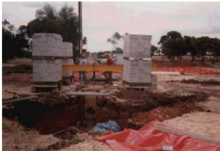
Figure 4-6. Reaction beam and dead weight system for loading the backfill surface of the buried pipes
