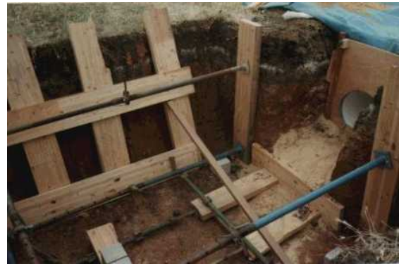
Fig 4-4d. End of pipe for monitoring of internal pipe displacements
